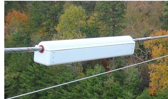
DSR Deployed on TVA 161 kV line
